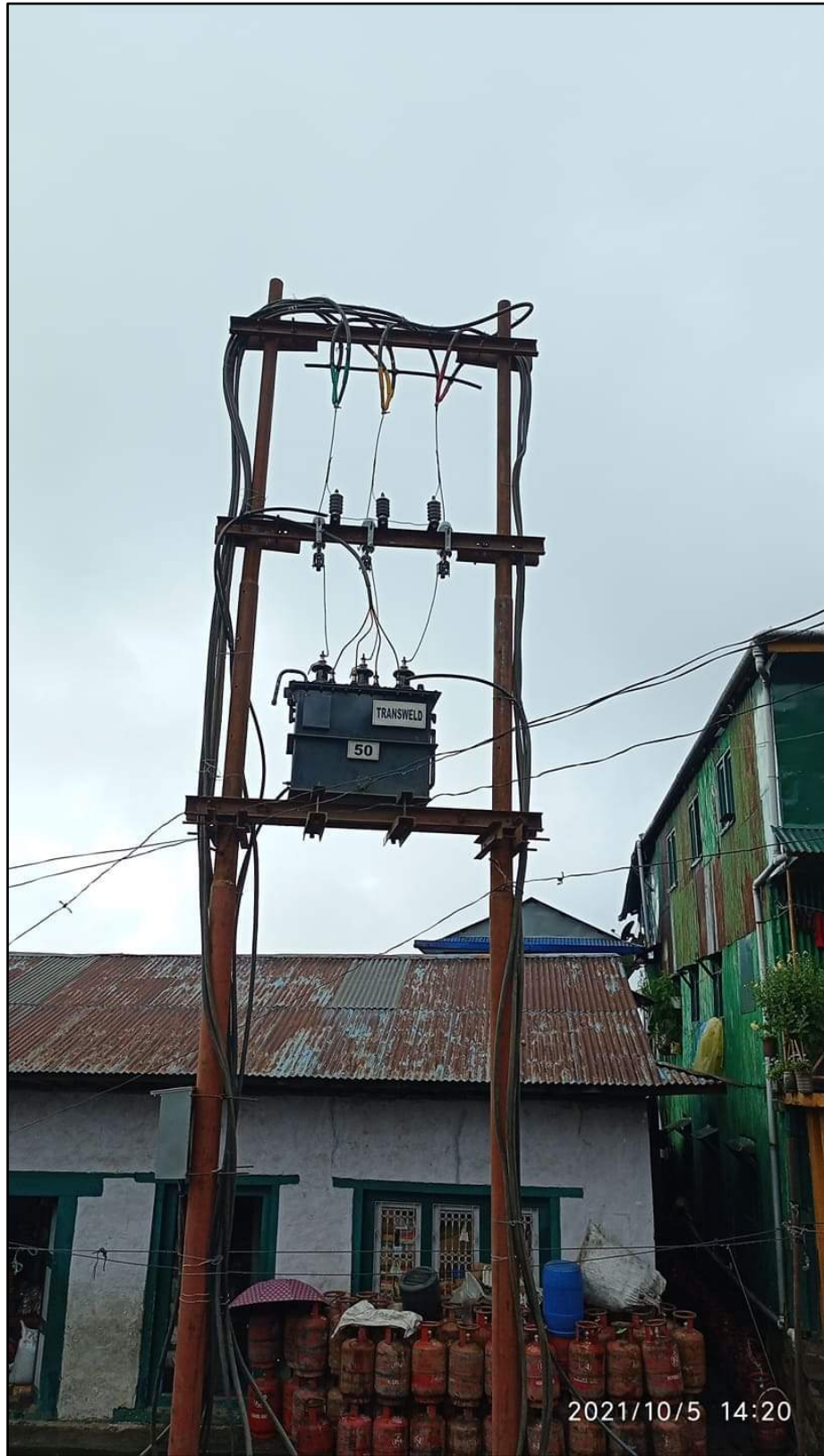
A Distribution Transformer in Lukla, Solukhumbu
