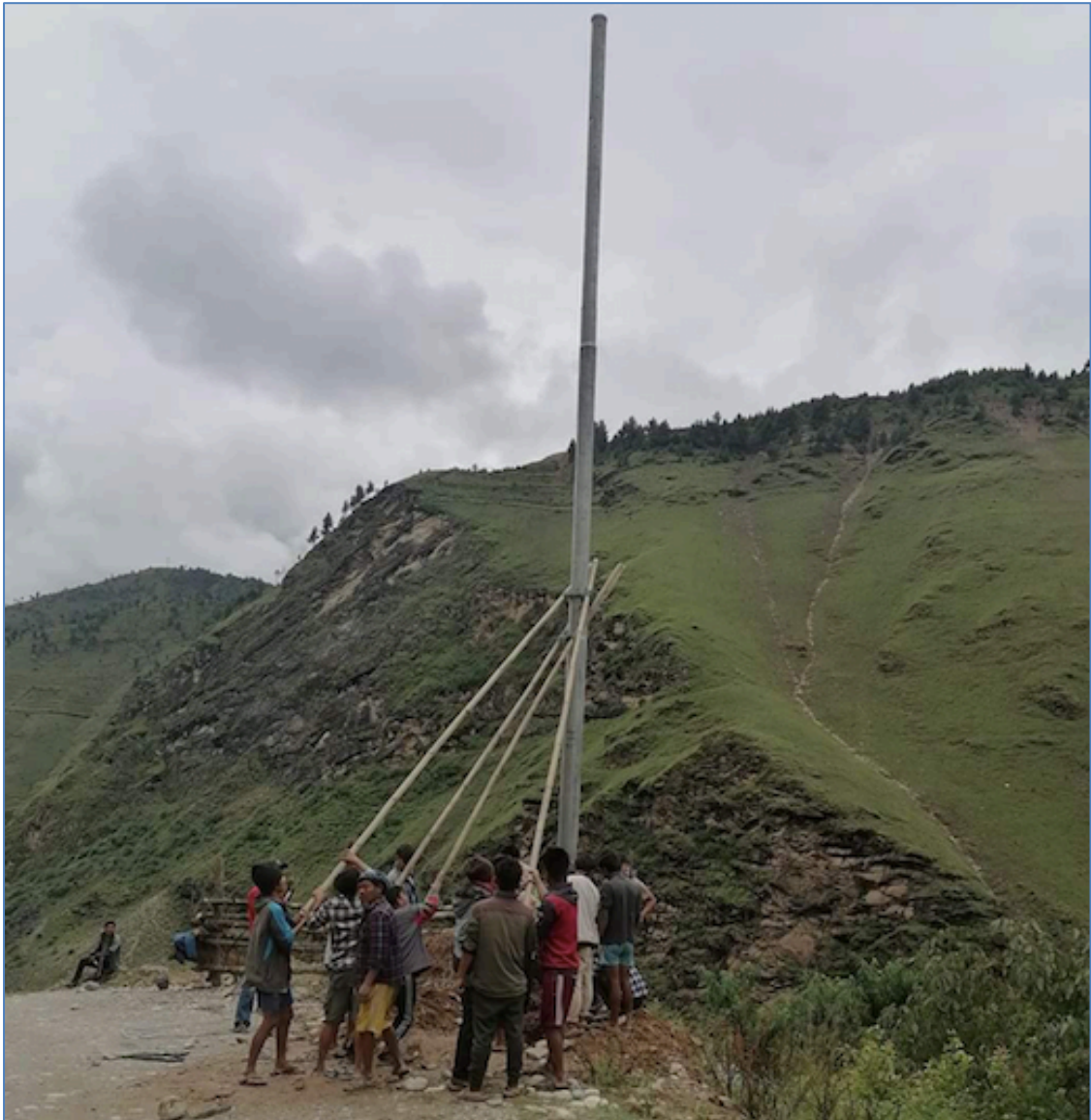
Transmission Line Distribution in Patarasi Chukeni Khola MHP, Jumla
